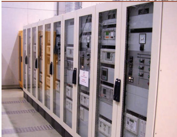
Control and protection equipment
